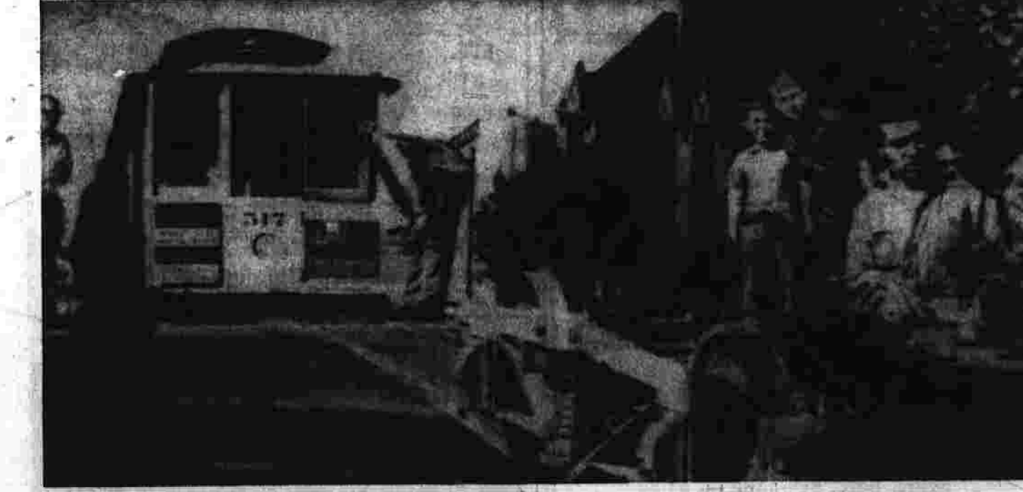
Workmen study problem of getting cable car back on its wheels after it took a dizzy ride in San Francisco. (AP Photofax.)
